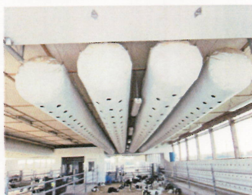
Wide barn – summer tubes and side wall ducts
