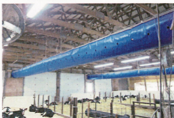
2 Cold weather tubes – 60 ft auto calf feeder barn
